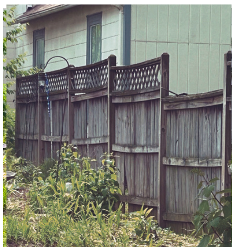
The old fence, in serious need of upgrade.
